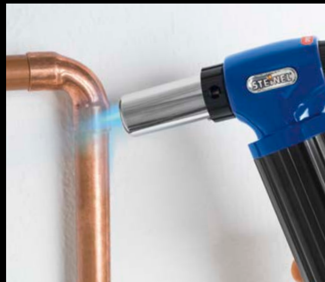
Solder joints on copper piping
